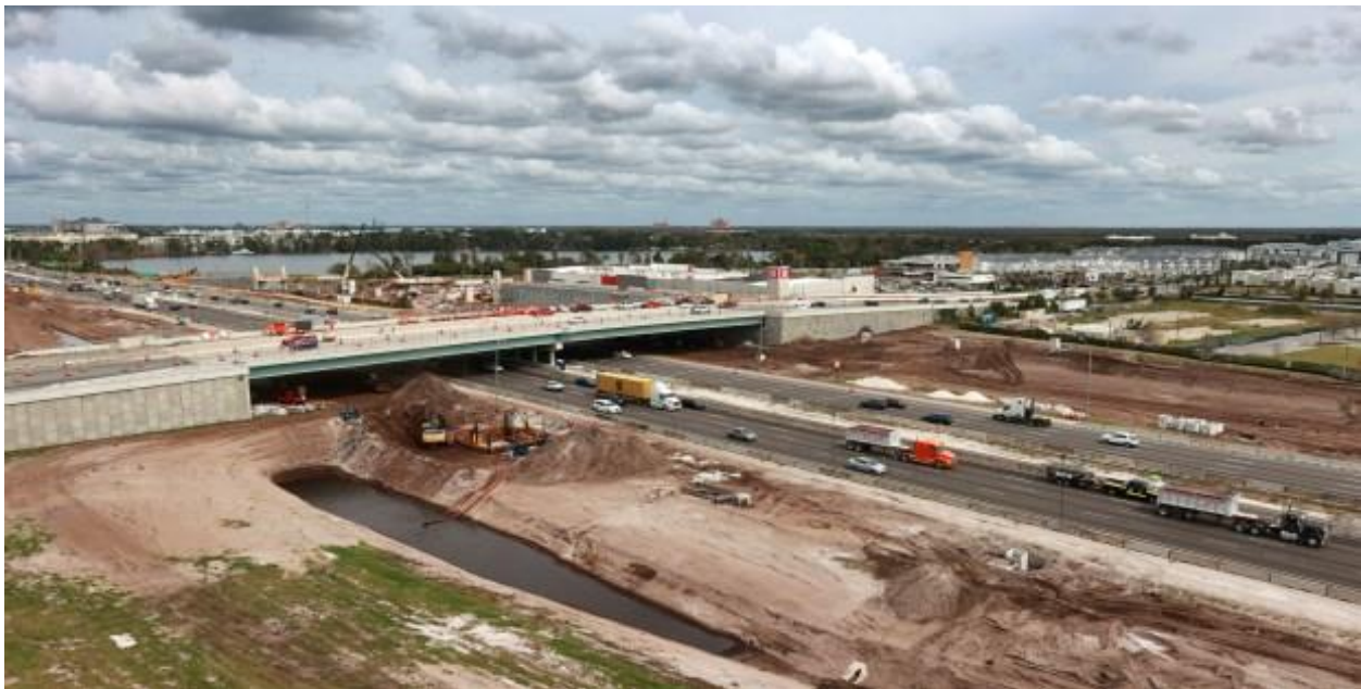
As seen from Daryl Carter Parkway near Disney Springs, construction continues on Interstate 4
